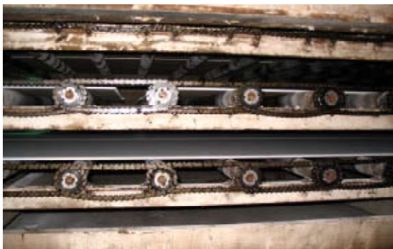
Conveyor line must constantly be lubricated and is replaced every 3 to 6 months.
